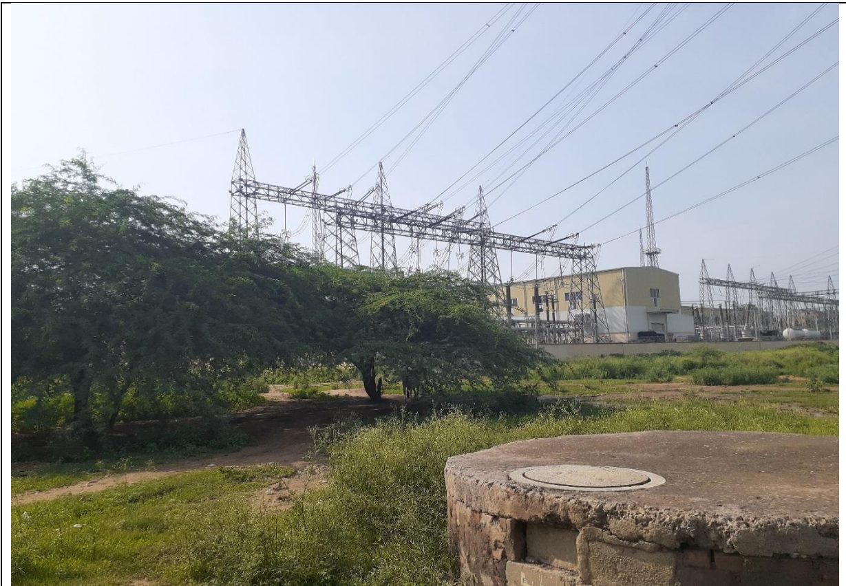
Photo 2 –Existing Sub Station of Power Grid Corporation at the Eco-sensitive Zone
